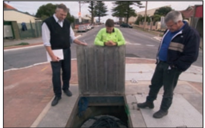
Alan Turner & John Nagel (Treliving Engineering) with Alan Chesters (Charles Sturt City Council) conducting a pit inspection.
